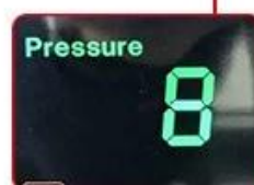
Internal pressure indicator in GY-08 controller
